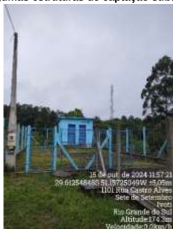
Poço CSB-61 (Wittmann)
